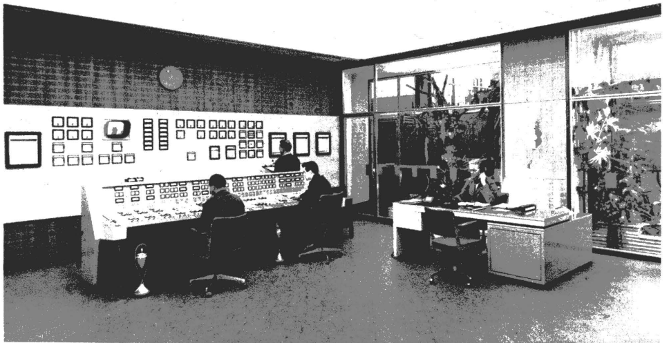
Bewag - Control room at the Oberhavel power station.
