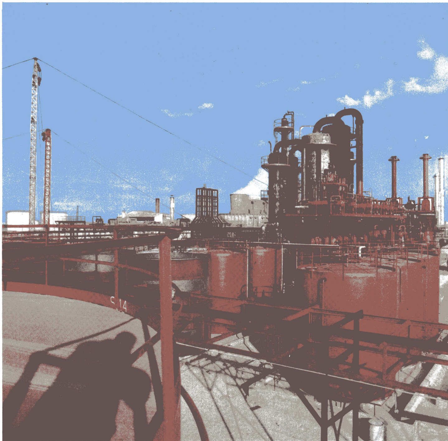
S.I.R. - Part of the plant.
