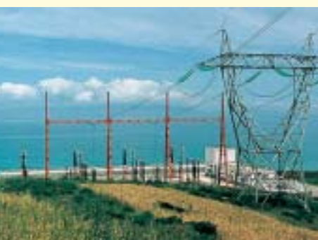
Power interconnection, Morocco
