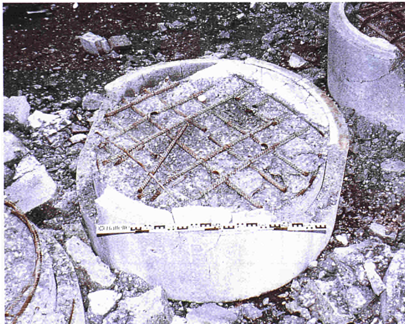
Figure 1: Comparison of concrete removal on test bodies of 1,4 m diameter a) exact simultaneous blasting b) sequential blasting
