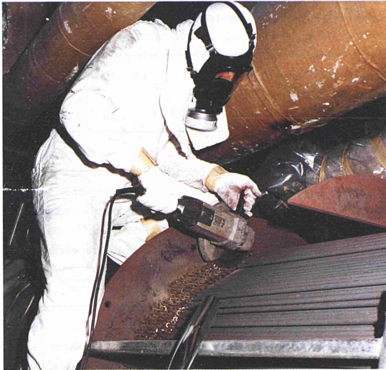
Fig. 1 - View of tube cutting works of the preheater No. 4 of Garigliano BWR.
