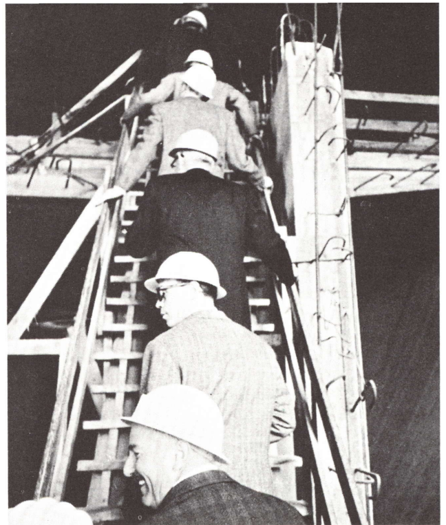
Inspection Tour: Euratom personnel view construction of the SENN project near Naples, Italy, which entered service during the year under the United States-Euratom Cooperation Agreement.
