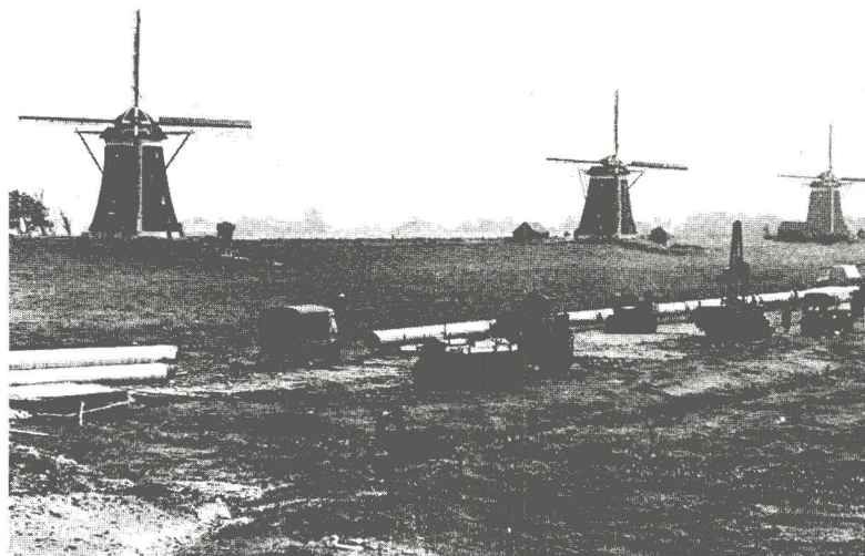
Installation of a pipeline in the Netherlands. Most of the necessary European pipeline network must still be installed.
