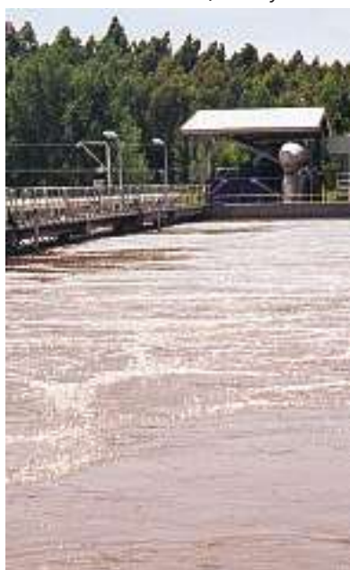
Water treatment Plant, Turkey
