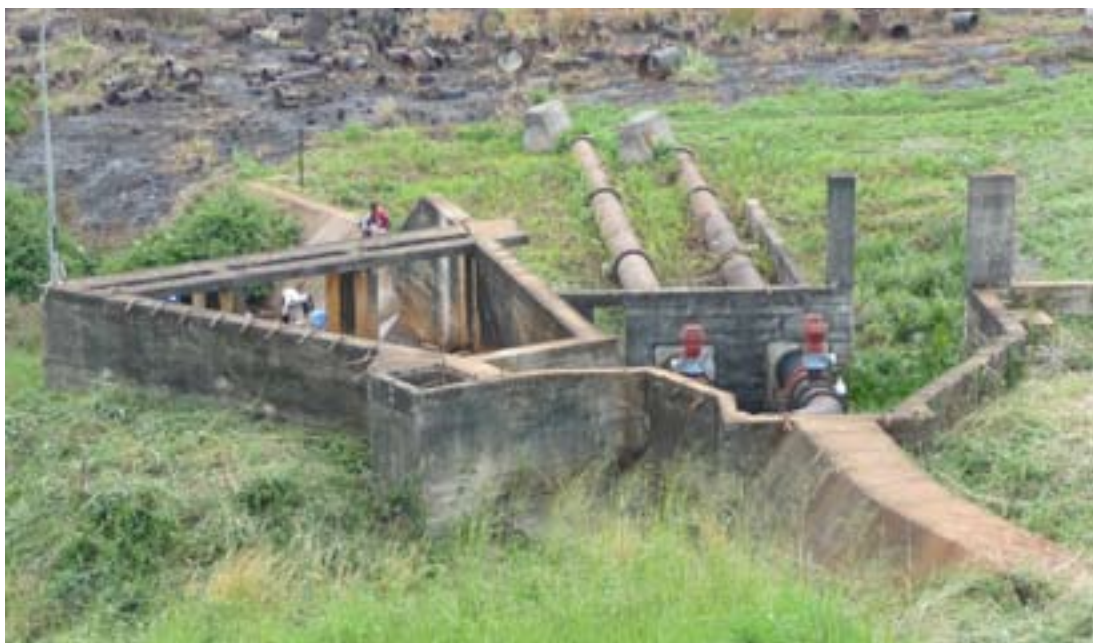
Bulk water pipes to be rehabilitated as part of the CAMWATER project
