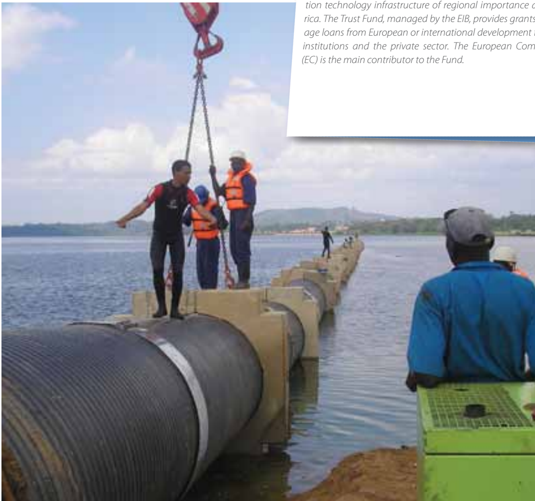
Gaba offshore pipeline, Kampala, Uganda
