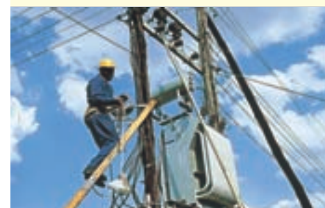
Modernisation of electricity grid
