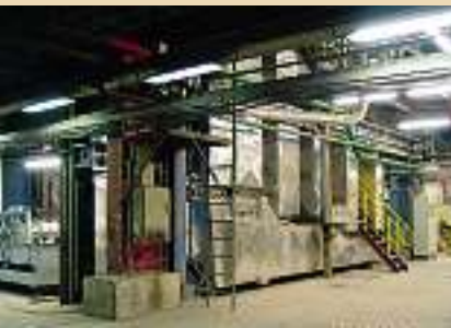
Waste incineration plant, Budapest
