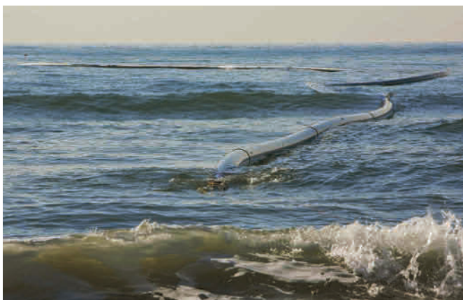
Submarine power cable, Italy
