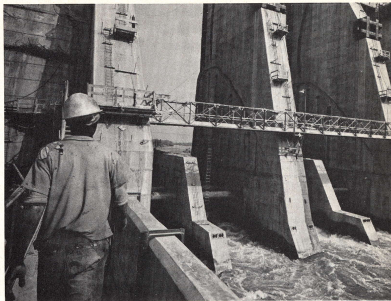
A hydroelectric project on the Niger River in Nigeria. World Bank photo by Yutaka Nagata
