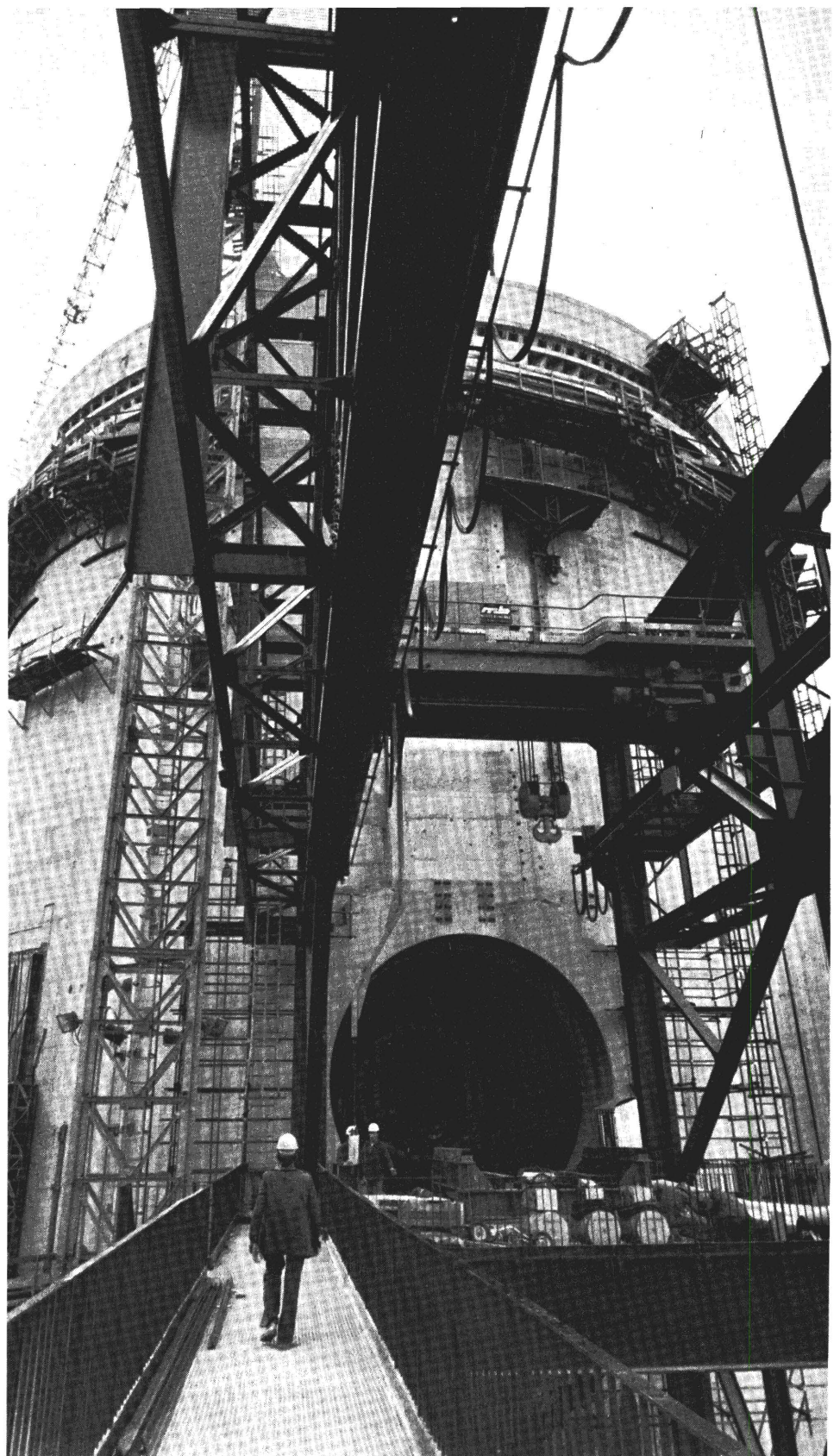
France has "notably the most audacious electro-nuclear program in the world." Shown here is part of the nuclear plant at Dampierre. © Black Star/Sipa Press
