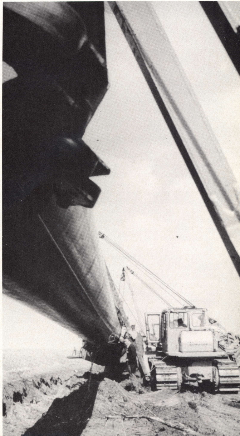
Construction of a gas main six years ago that will be connected with the new Siberian pipeline. © TASS from Sovfoto, New York
