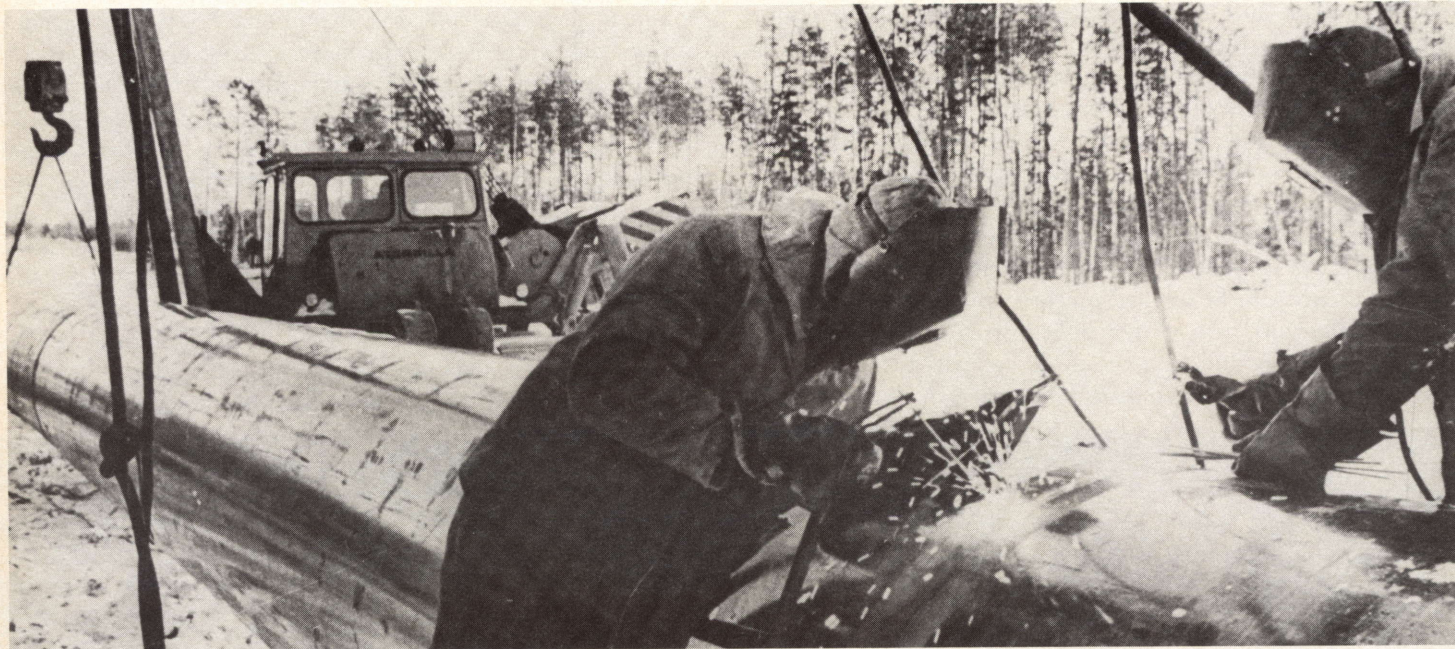
Construction on the Siberian gas pipeline, the center of last-year's dispute between the Americans and the Europeans over the application of U.S. laws to foreign-based subsidiaries and licensees of U.S. firms. © Sygma
