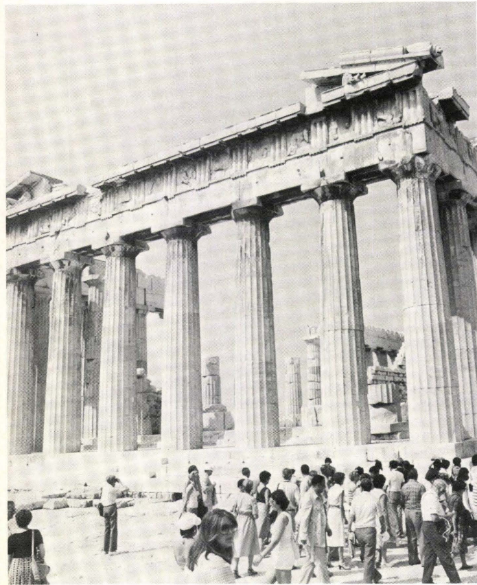
Major restoration is currently underway on the Parthenon to prevent further decay and restore its former beauty.
