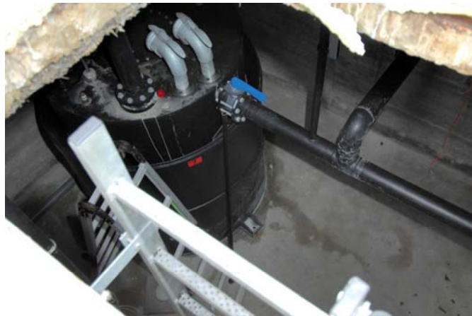
Waste water tank
