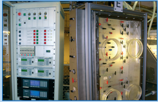
Figure 31 - Instrumentation cabinets and control panels of the extension of the Tritium Measuring Station at HFR, applied for irradiation experiments with tritiated purge lines
