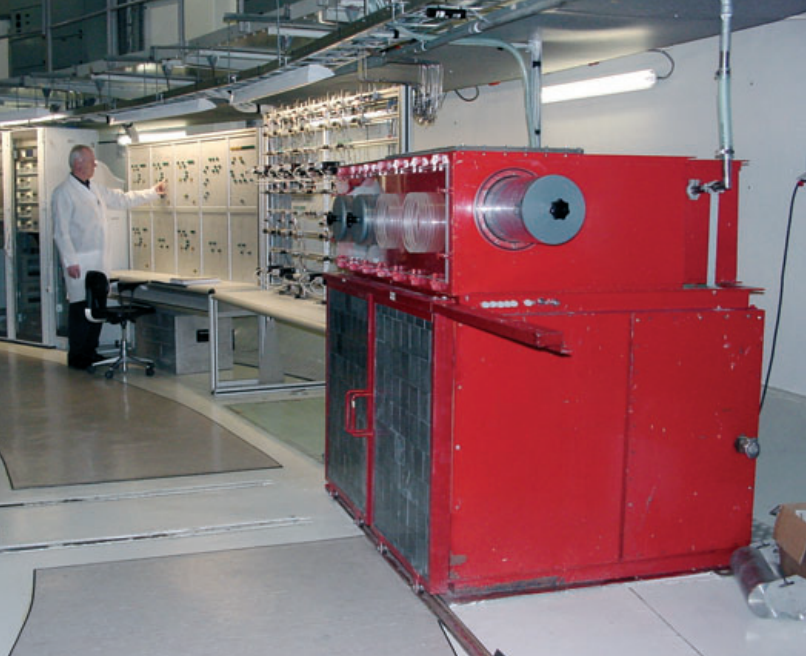
Figure 25 - Sweep Loop facility installed in the HFR basement
