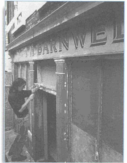
The Dublin project, "Maintaining the Historic Heart of Dublin", not only envisages the creation of a database inventory of pre-1900 buildings, but will also produce manuals concerning the maintenance of historic buildings. The project will also refurbish three historic buildings as demonstration projects, to encourage further restoration activities in the area.
