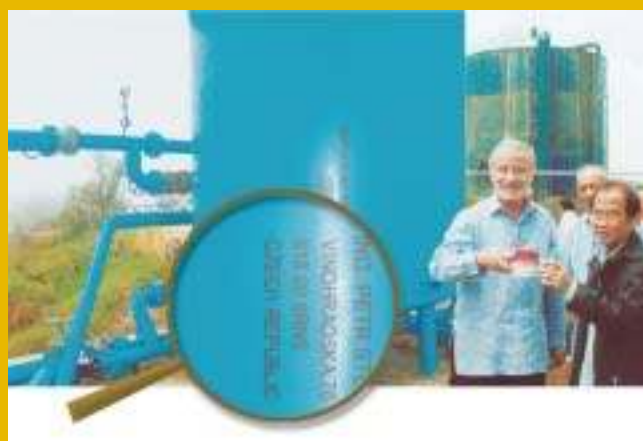
Czech Republic Development Assistance to the Philippines includes the supply and commissioning of three water treatment plants and pressure water filters in Baguio City. The water treatment plants were installed on three sites of the Baguio Water District. (Photo Credit: Embassy of the Czech Republic)
