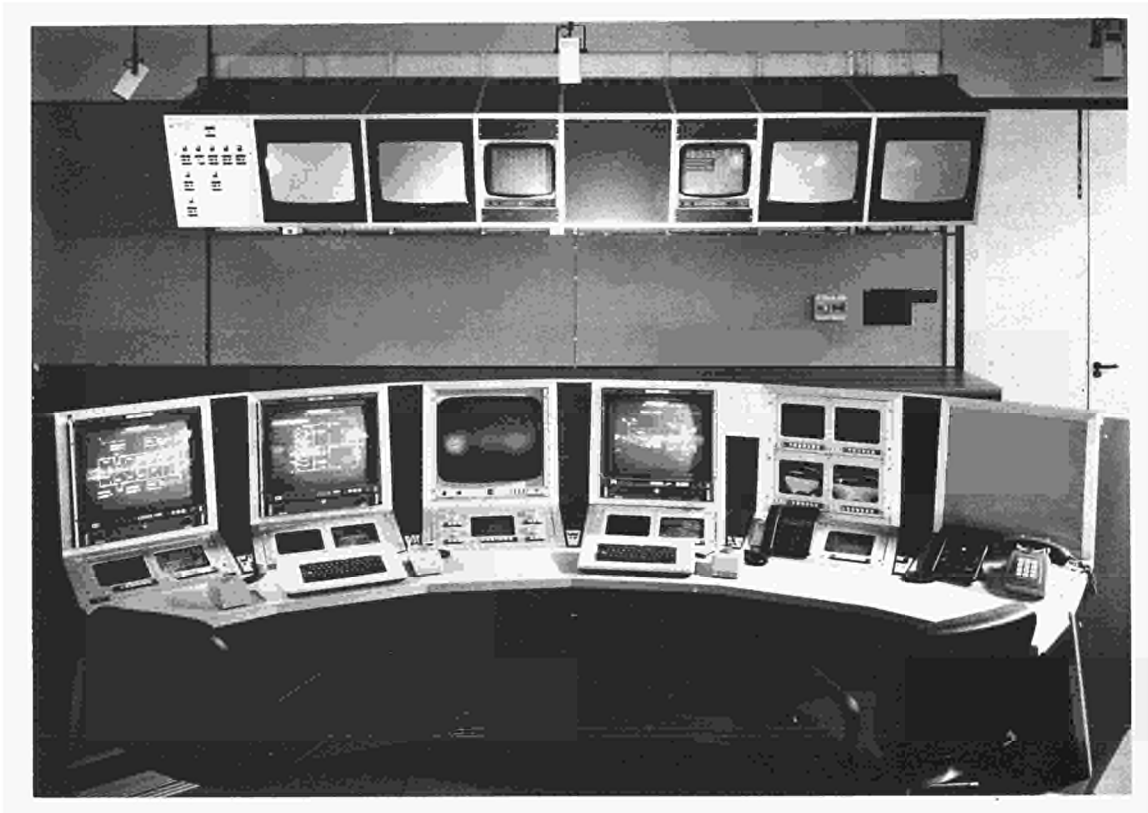
Fig. 31 JET Machine Control Room Console with Synoptic view above.
