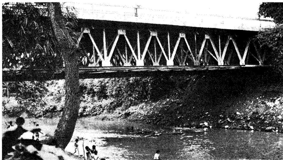
Photo 4 A four lane Callender-Hamilton Type B deck Bridge in Indonesia. This structure can be simply up-graded as traffic flows increase by the addition of extra trusses. See section 3.7
