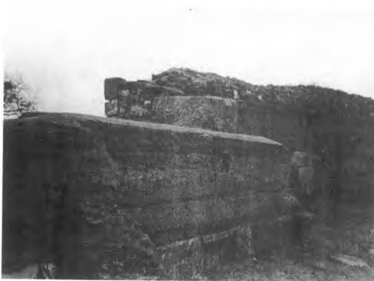
Fig. 3 Damage and deterioration of the stone
