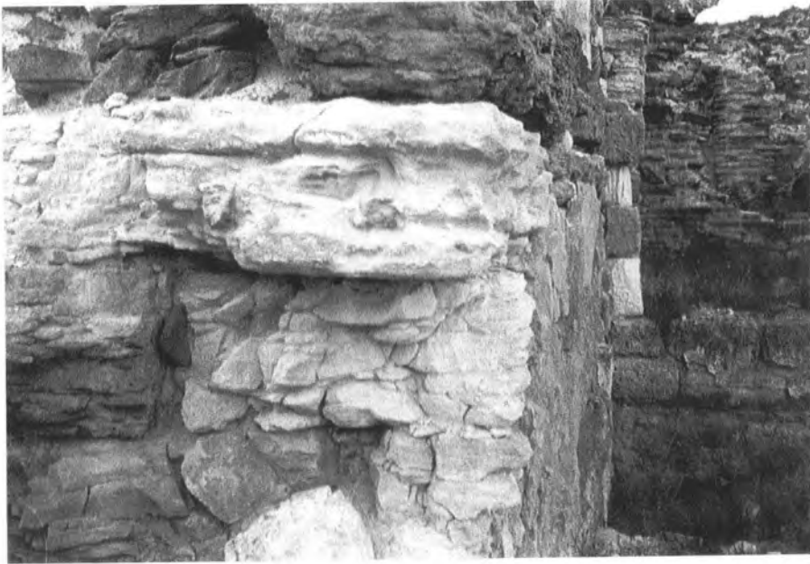
Fig. 4 Damage and deterioration of the stone
