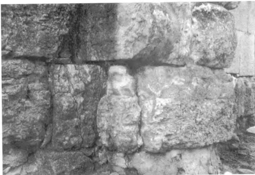
Fig. 5 Damage and deterioration of the stone
