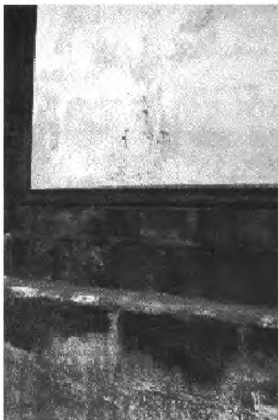
Fig. 8b Detail of the left corner of the façade with evidence of efflorescences on both the skirting board and the plaster
