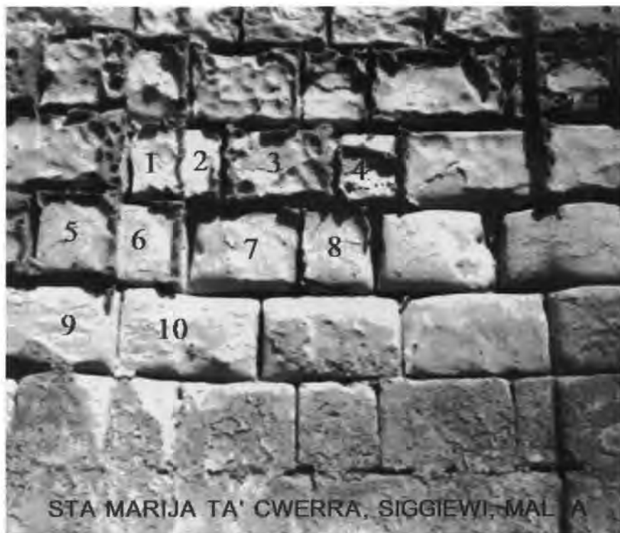
Fig. 6 A part of the external southern wall of the church. Numbers correspond the points of measurements.
