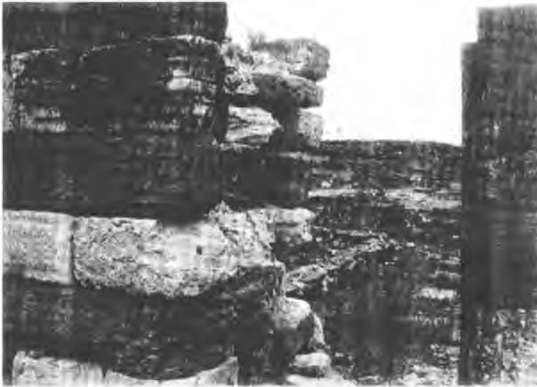
Fig. 8 Damage and deterioration of the stone
