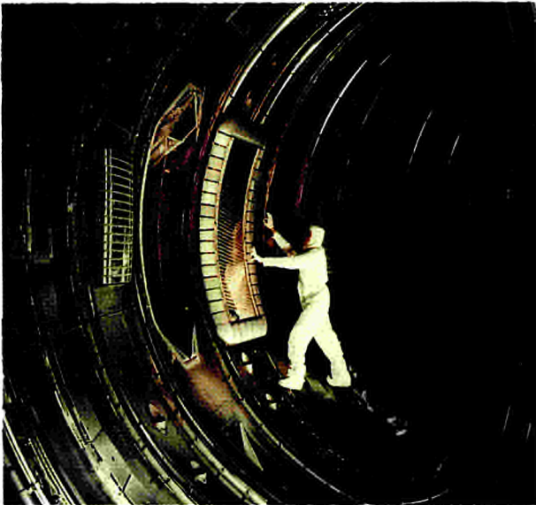
Fig. 25 An RF antenna and limiters mounted on the interior of the vacuum vessel.
