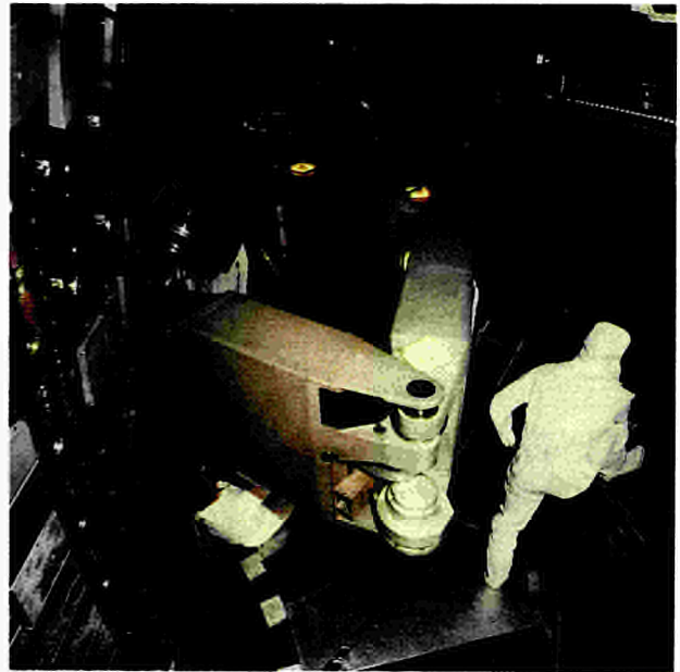
Fig. 23. The articulated boom being used to install sections of the belt limiter.
