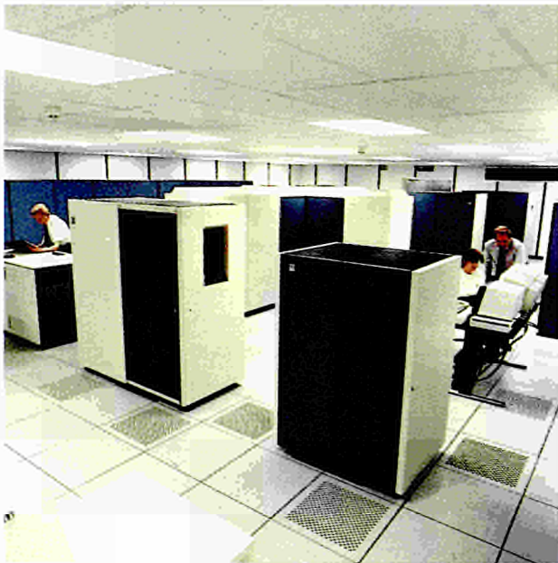
Fig. 19 The new JET mainframe IBM Computer located at Harwell
