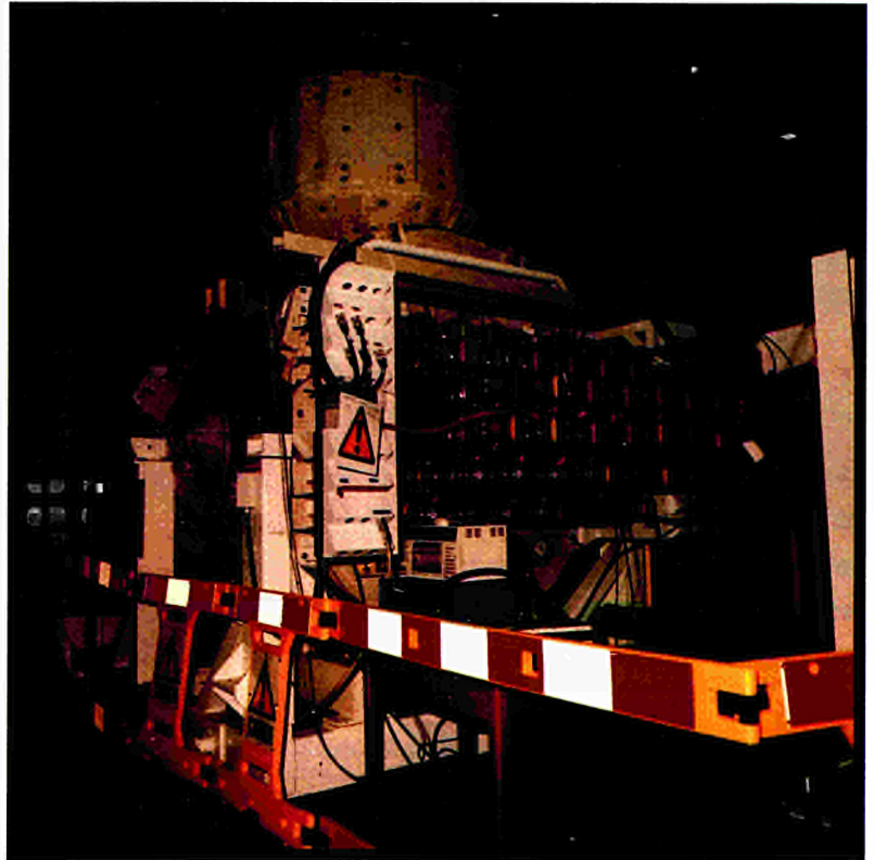
Fig.29: A view of the forty-eight vacuum windows connecting the LHCD waveguides to the rear of the launcher.
