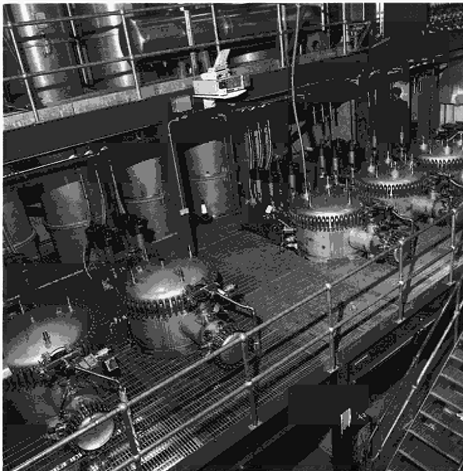
Fig.200: View of the Active Gas Handling System showing the five cryogenic forevacuum modules with buffer tanks and cryodistribution system in the background.
