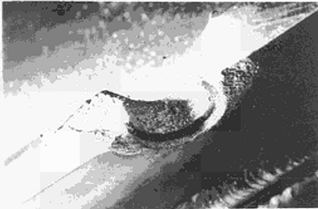
Fig. 4: Damage to bellows protection plate fixing slot caused by arcing.
