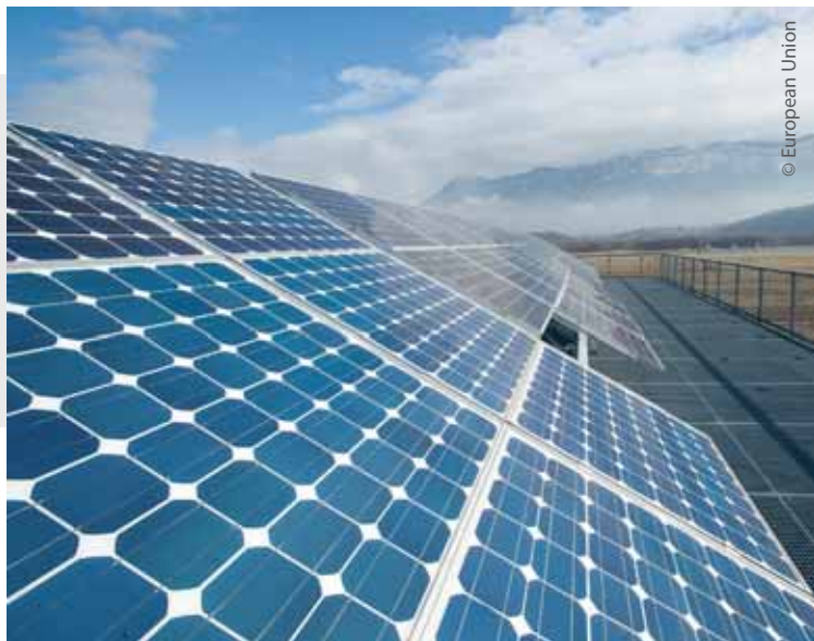
Solar panels in France
