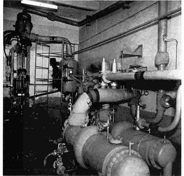
Loop for large-scale heat-transfer tests, installed at Genoa.
