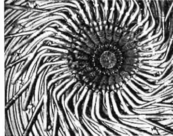
Inside the AVR pebble-bed reactor in Jülich: a heat-exchanger.
