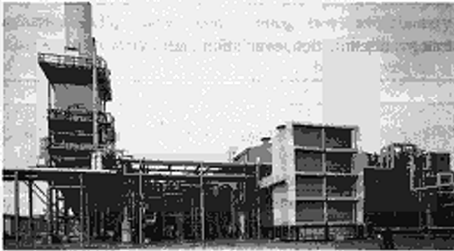
Air intake assembly of a gas turbine plant with modified heat recovery boiler
