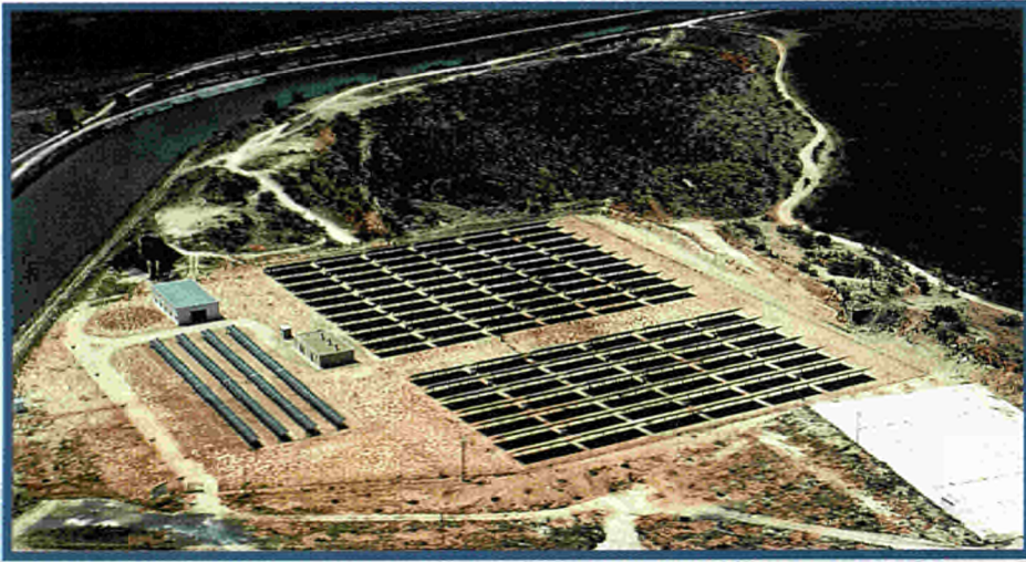
A 1MW photovoltaic power plant in Toledo (Spain), established with THERMIE support.
