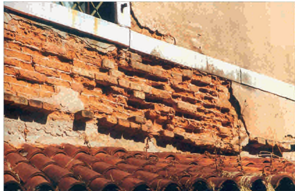
Venice: salt damage to brickwork and plaster.
