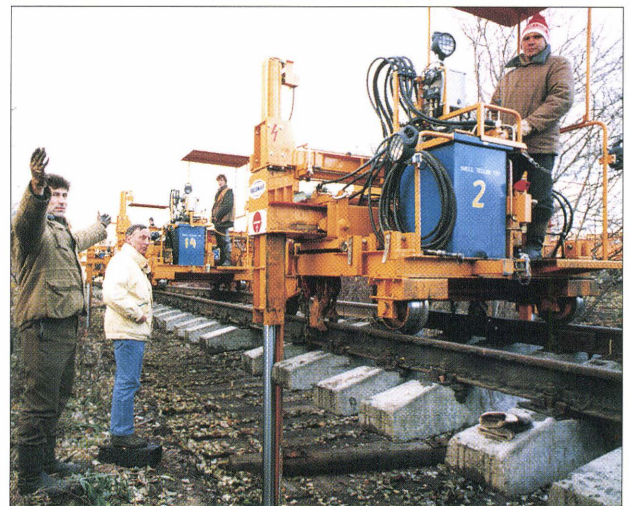
Training machine operators and future trainers from the October Railway in light track maintenance: replacing a track panel and switchgear
