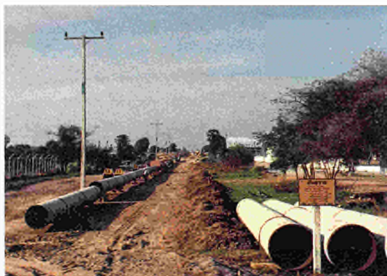
Energy infrastructure ranks at the forefront of EIB lending in the ALA countries
