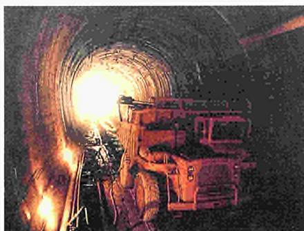
Key EIB objectives range from financing large infrastructure to supporting small and medium-scale productive investment
