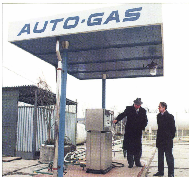
Making life easier for motorists - an LPG filling station in working order.
