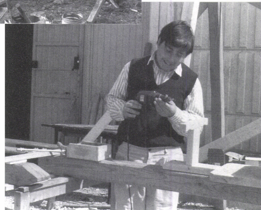
Building of an open-air playground by people with mental health problems, reflecting their many vocational abilities (LMA Rieti / It)
