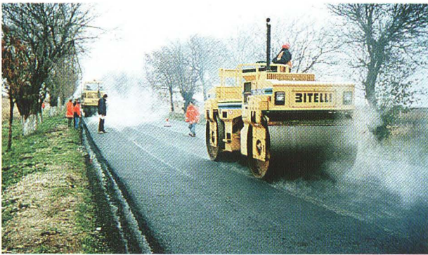
Budapest - Gyöngyös motorway in Hungary, the Via Baltica in Lithuania and sections of the Ljubljana - Celje motorway in Slovenia.
