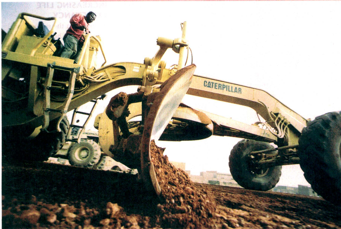
Burkina Faso. Construction of the Bobo-Dioulasso road in the direction of Mouni.
